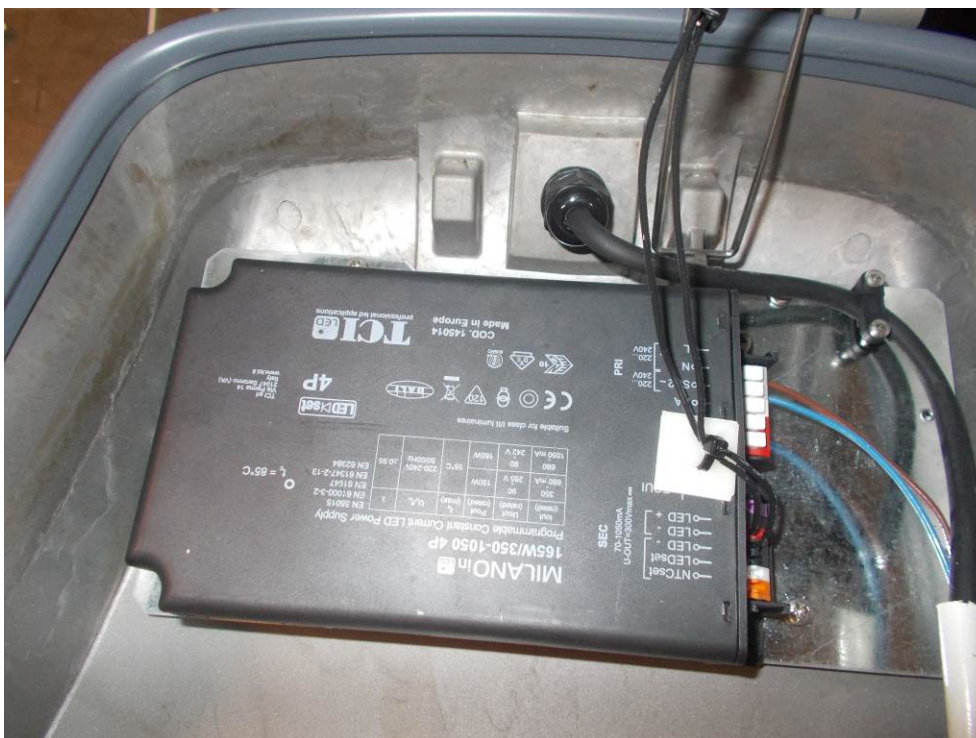
Pic.8: internal view
